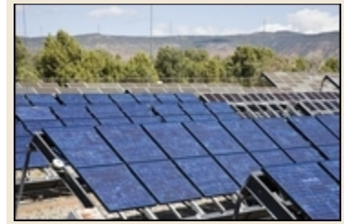
Hoku Solar's 12-acre solar farm would rank among the U.S.'s largest.
